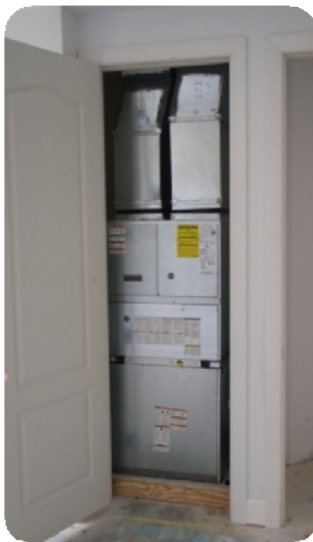
Figure 5: Magic-Pak HVAC unit in Bedroom
